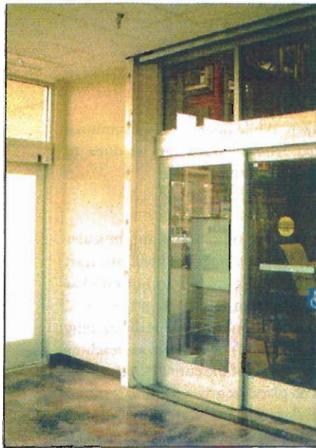
Left: Aesthetically pleasing flood-proofing. The gate is stored in a false ceiling and can be lowered into place in minutes.
