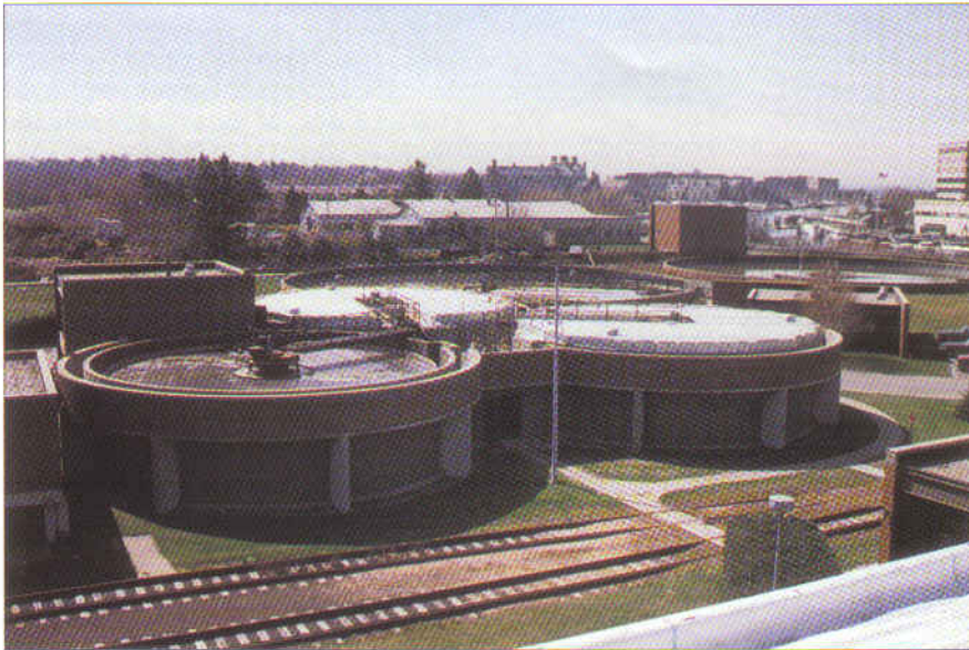
Flat covers on wastewater plant process tanks contain the odors and gases generated in them but are an unobtrusive addition to the facility.
