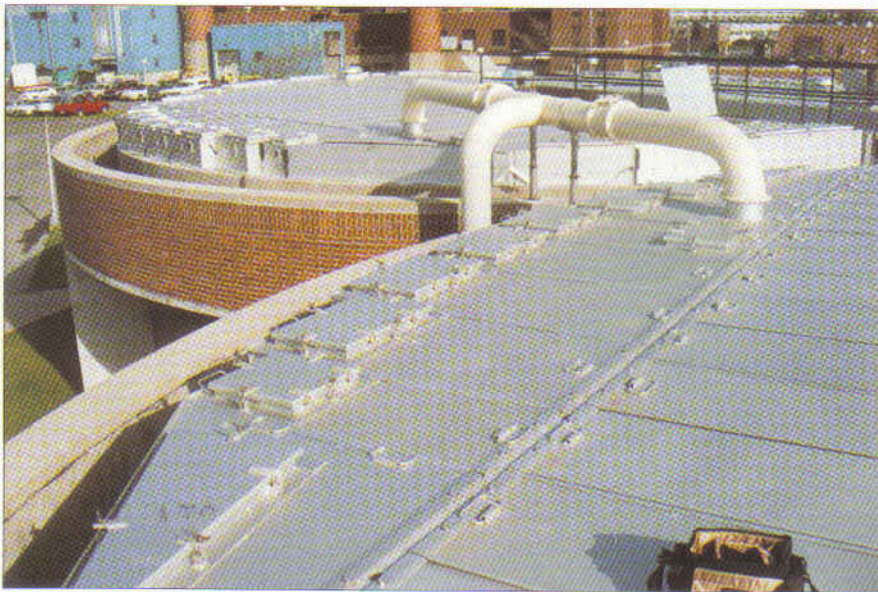
Close-up of flat covers shows the modular fabrication style of these systems, and the ports which allow operator access to selected equipment or process areas.
