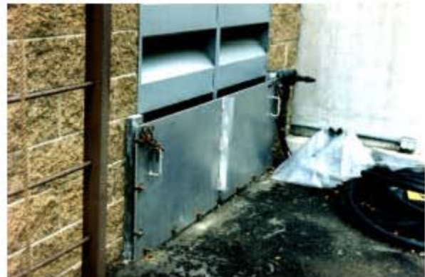
VENTS ARE OFTEN OVERLOOKED AS POINT OF ENTRY OF FLOOD WATER
