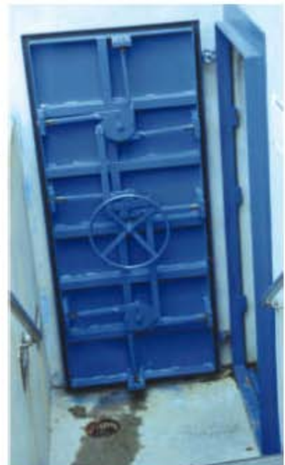
BELOW GRADE BASEMENTS - ELECTRICAL ROOMS, ELEVATORS CAN BE PROTECTED WITH WATERTIGHT DOORS
