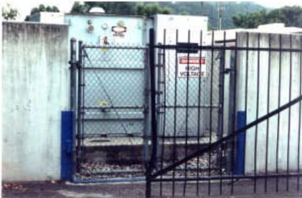
ELECTRICAL VAULT IS SECURED BEHIND A FLOOD WALL WITH REMOVABLE FLOOD PANELS PROVIDING BOTH PROTECTION AND ACCESS
